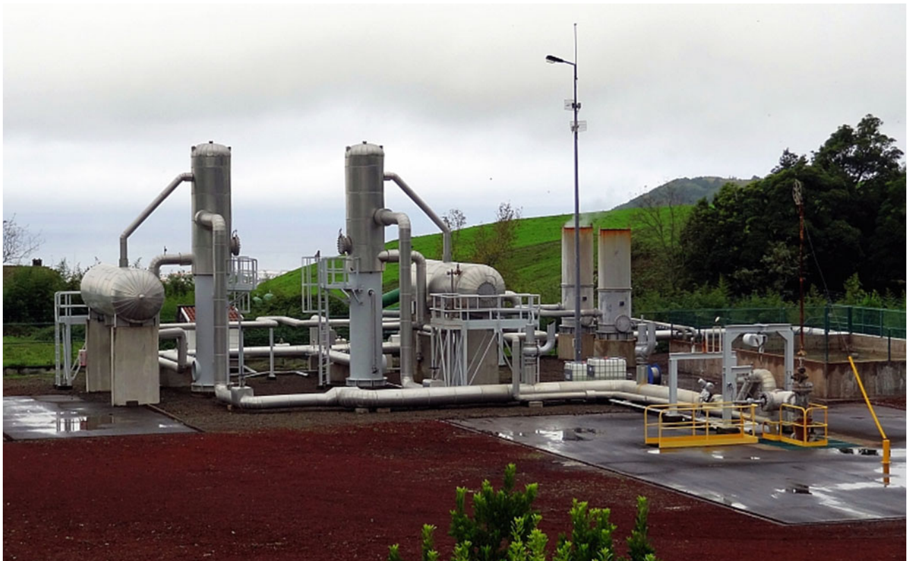
Fig. 11.5 Geothermal power plant in Terceira, one of the nine islands of the Azorean Archipelago
