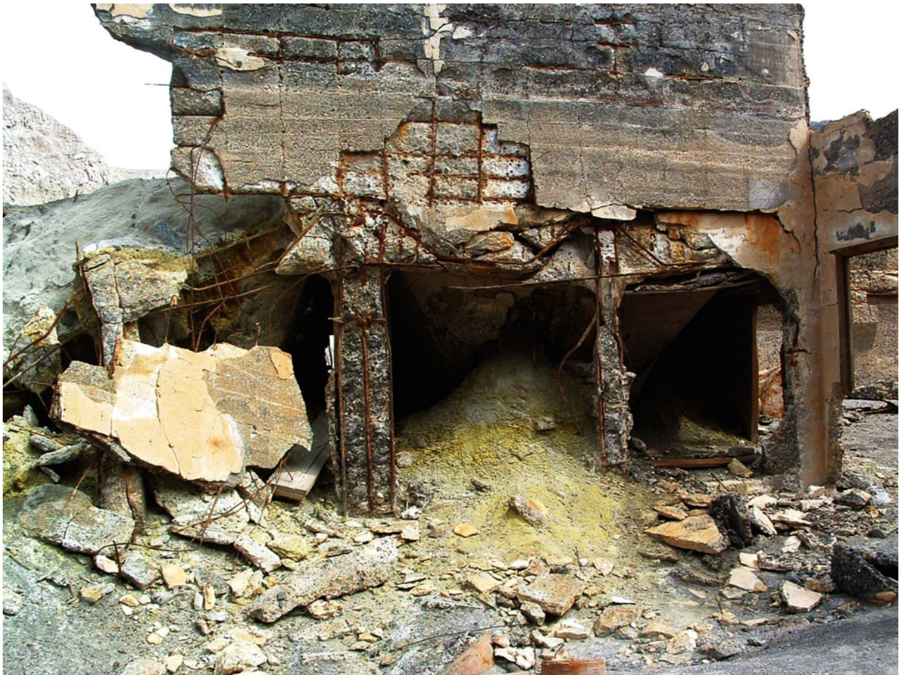
Fig. 2.11 Remnants of the destroyed sulphur mining facility on White Island approximately a decade ago. Prolonged exposure to acidic gas emissions from the nearby crater and occasional eruptions have further damaged the structure over time
