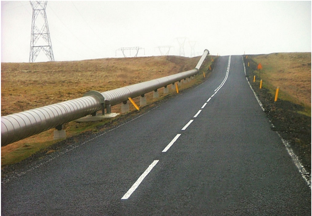
Fig. 11.3 This insulated steel pipeline is 27 km long and has the capacity to carry up to 1850 L per second of 100 °C hot water from the Nesjavellir geothermal power plant (Hengill high-temperature field) to storage tanks in Reykjavík (Iceland)
