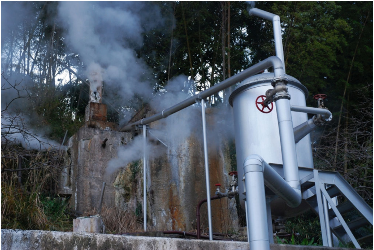
Fig. 3.15 Communal hot spring water supply is common in areas rich in hydrothermal resources. Due to extreme mineralisation, new installations are added to deteriorated and weakened older hot water tanks (Kyushu, Japan)
